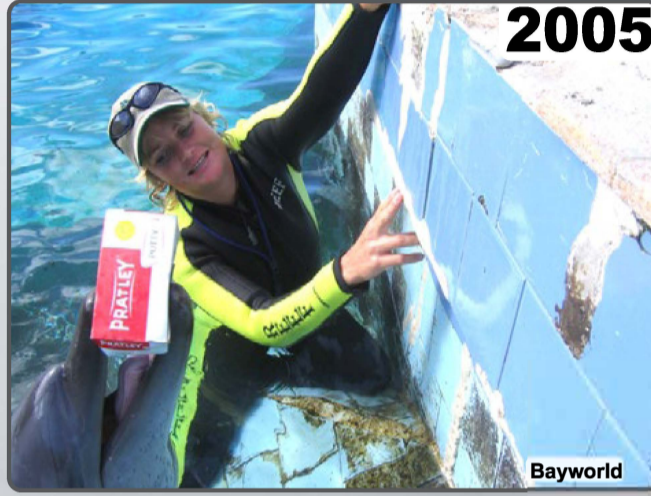
Pratley Putty was used to extensively repair areas of broken tiles of the Bayworld Aquarium tank in Port Elizabeth.
