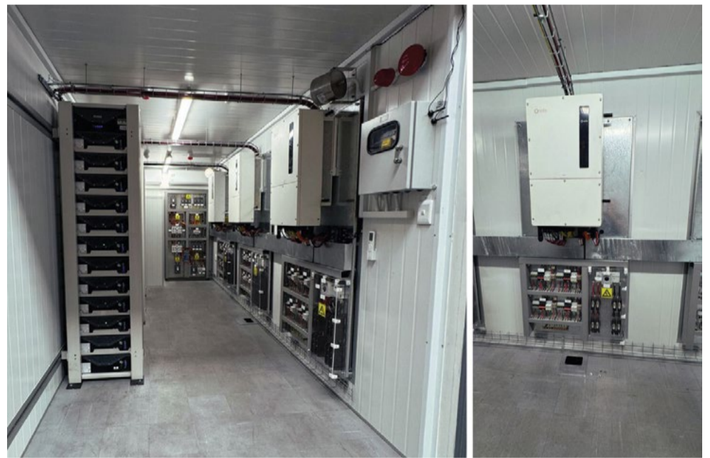
The BESS container.
