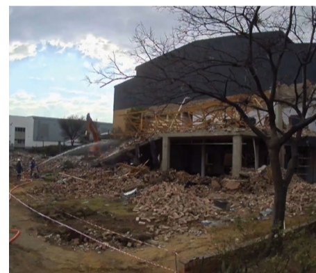
Initial demolition and site construction took six months, with the final fitting taking place in April 2024.
