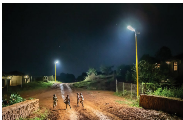
The solar-powered streetlights on GRP poles create a safe environment for women and children, and pedestrian visibility at night.
