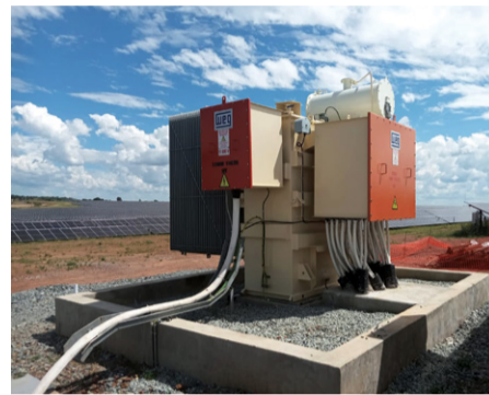
The MV and LV terminal boxes of the 5 MVA PV transformers.
