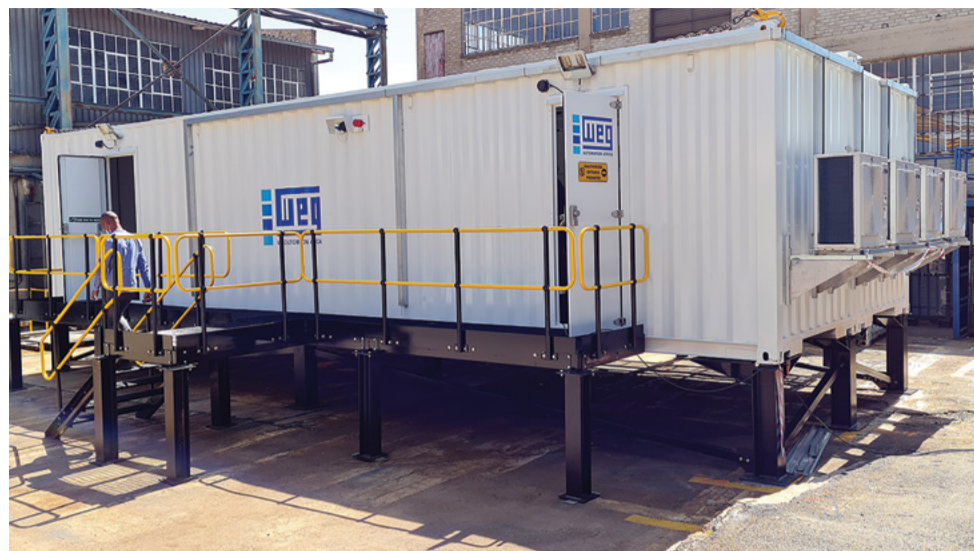
The double containerised electrical house.
