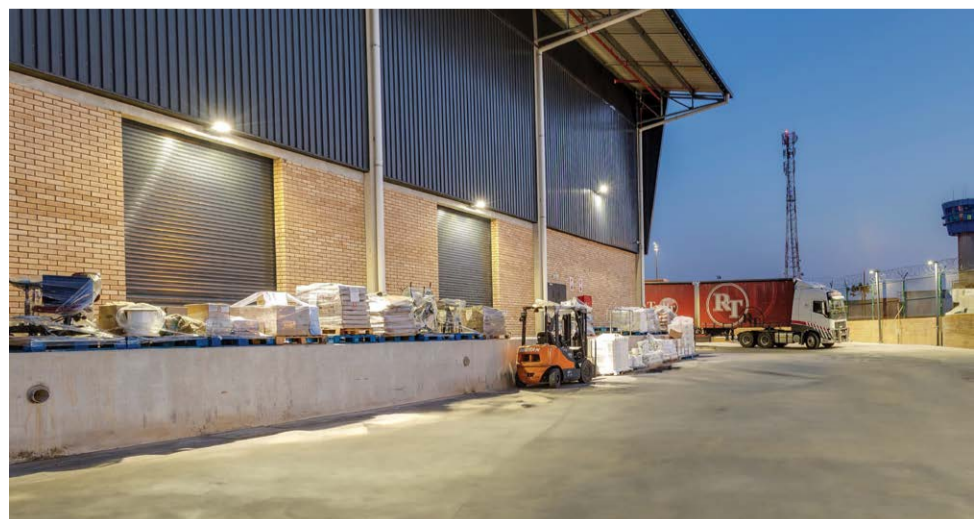
BEKA Schröder's LEDLUME and ELLEGA luminaires have been installed to provide area lighting.
