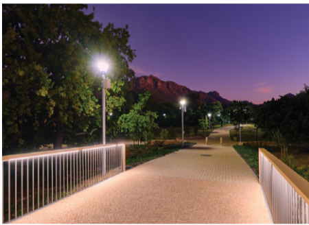
BEKA Schröder has supplied a complete smart lighting solution for a public walkway in Stellenbosch
