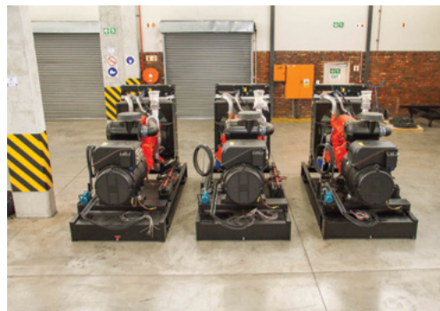
Generators at the Zest WEG manufacturing facility in Cape Town.
