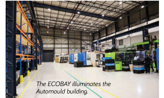
OMNISTAR-MAXI highbays illuminate the manufacturing plant and warehouse in the Sodecia Cluster.
