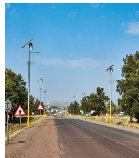
BEKA SOLAR streetlights have been installed throughout Postmasburg.
