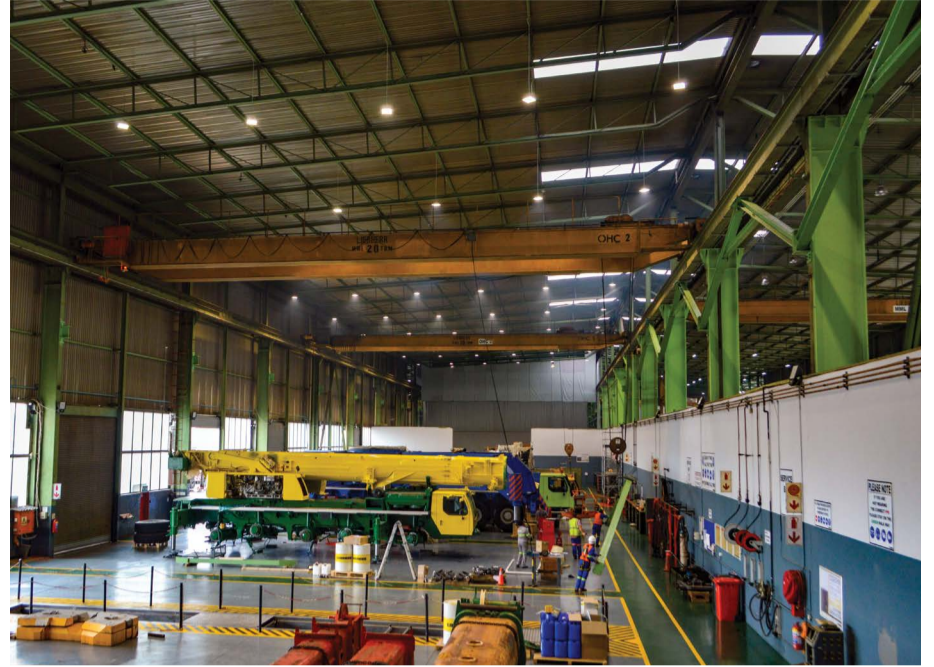
The locally designed and manufactured ECOBAY illuminates Liebherr-Africa's crane workshop.
