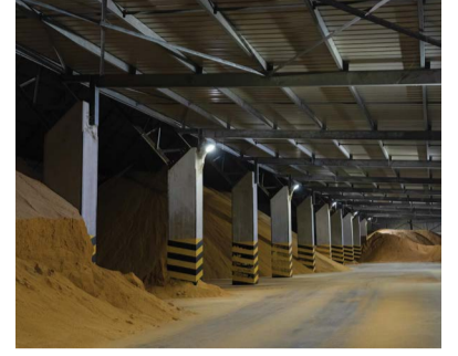
The OMNISTAR-MIDI has been installed in the grain offloading area.
