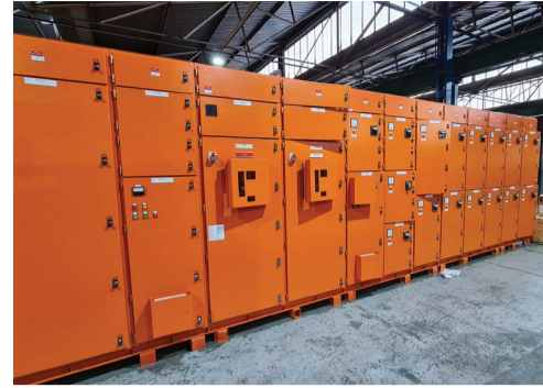
Motor control centres at Zest WEG's manufacturing facility in Robertsham.
