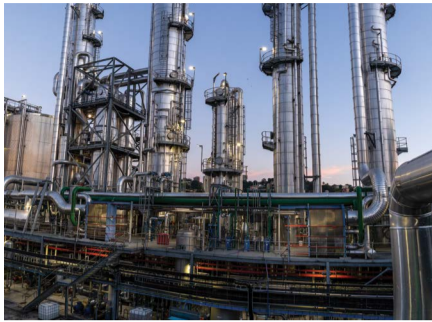
BEKA Schröder has supplied the LED lighting solution for AlcoNCP in Durban.
