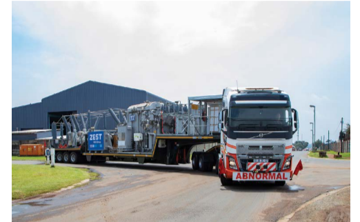
Zest WEG will showcase its mobile substation capabilities at Electra Mining
