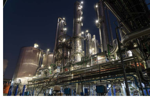
The LEDNOVA-MIDI and BEKA VAPOURLINE are suitable for Zone 2 applications were installed throughout AlcoNCP's distillery.
