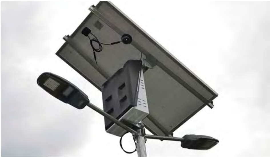
With the solar-powered luminaires, visibility at night is increased, and a child-friendly environment for the community children as well as the neighbouring schools is created.
