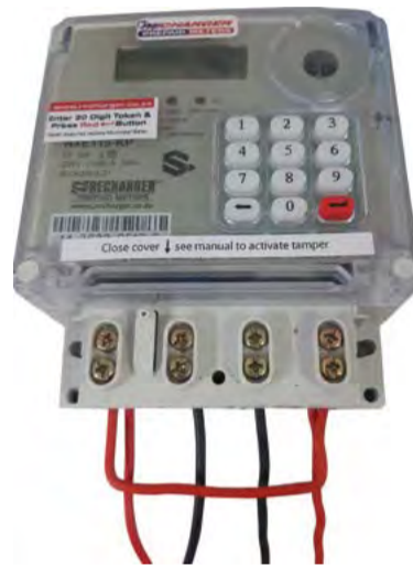
Illegal bridge connection.
