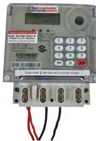
Illegal bypass connection.
