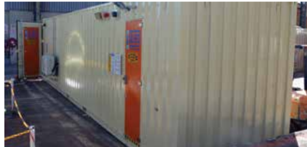
A 12 m containerised substation housing WEG Automation Africa IEC61641 internally arc tested fixed pattern Motor Control Centre.
