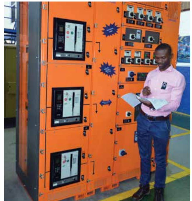
A fully withdrawable IEC61439 and IEC61641 compliant Motor Control Centre manufactured at WEG Automation Africa.
