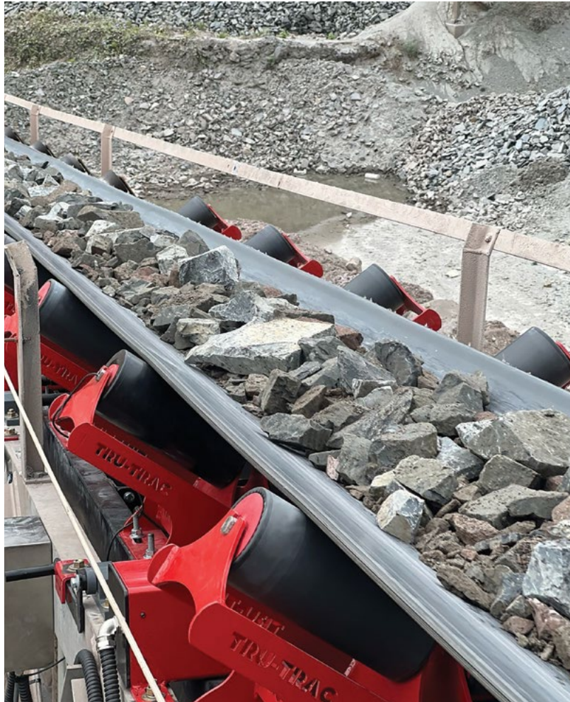
Tru-Trac belt scales installed in harsh industrial conditions, demonstrating their durability and reliability.
