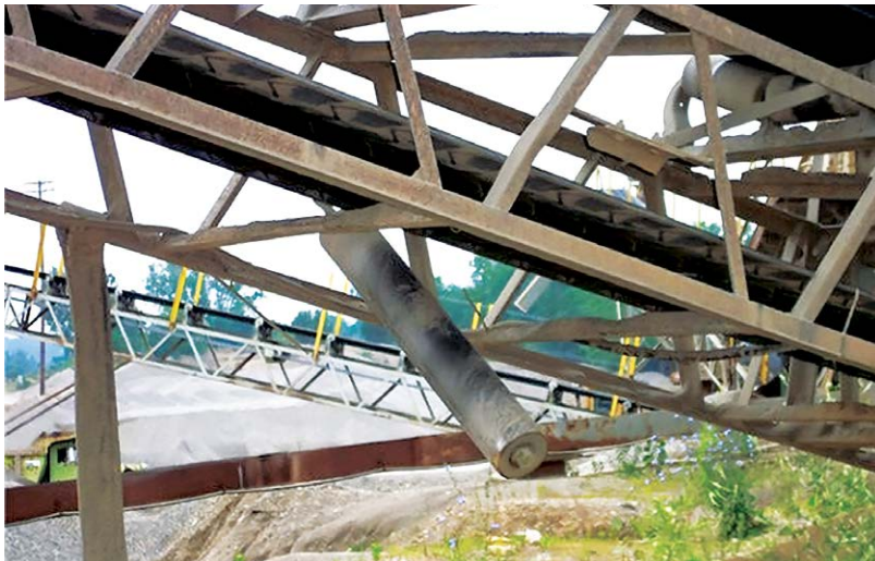
Unguarded return rollers over walkways can fall and produce a serious hazard.
