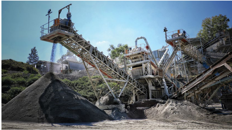
The oversized parts of the aggregate get sent back to a 36 inch Osborn crusher. The G5 is deposited onto a stockpile while G2 material goes through a vertical shaft impact crusher and then to the stockpile.
