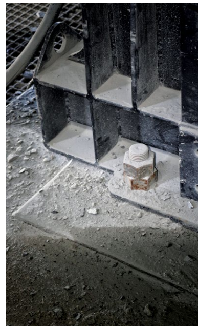
The new C120 Metso crusher that replaced the previous crusher is now mounted on dampers. The dampers reduce the dynamic forces from the crusher onto the support steel – almost like shock absorbers.
