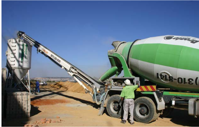
Some readymix concrete companies can offer specially designed delivery vehicles that incorporate either a concrete pump or conveyor.
