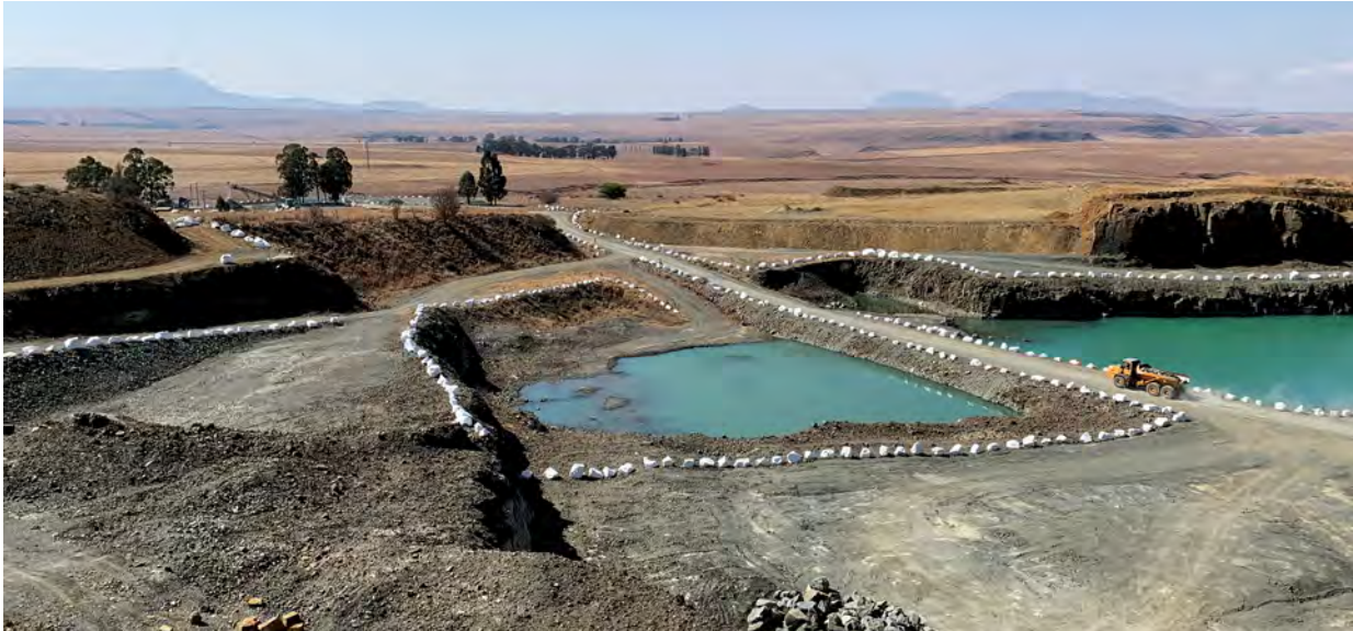
Traffic management on site is a crucial aspect of the safety regime on site.
