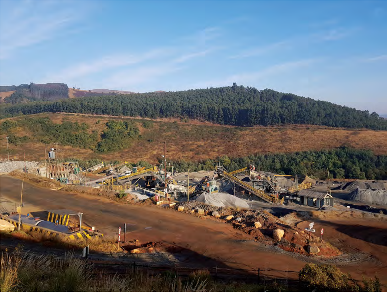
Midmar Crushers has over the years invested in several capital projects to improve processes on site.
