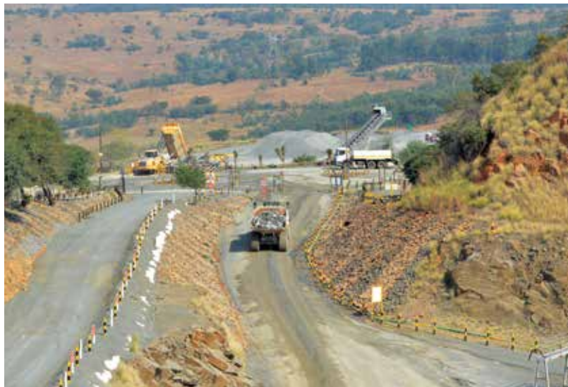
Traffic Management was one of the focus areas for the ISHE Audits during 2019.
