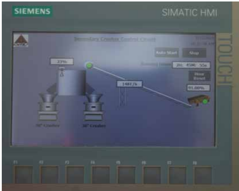
A Siemens PLC has been installed on the circuit to automatically regulate the feed box at the secondary crushing plant.
