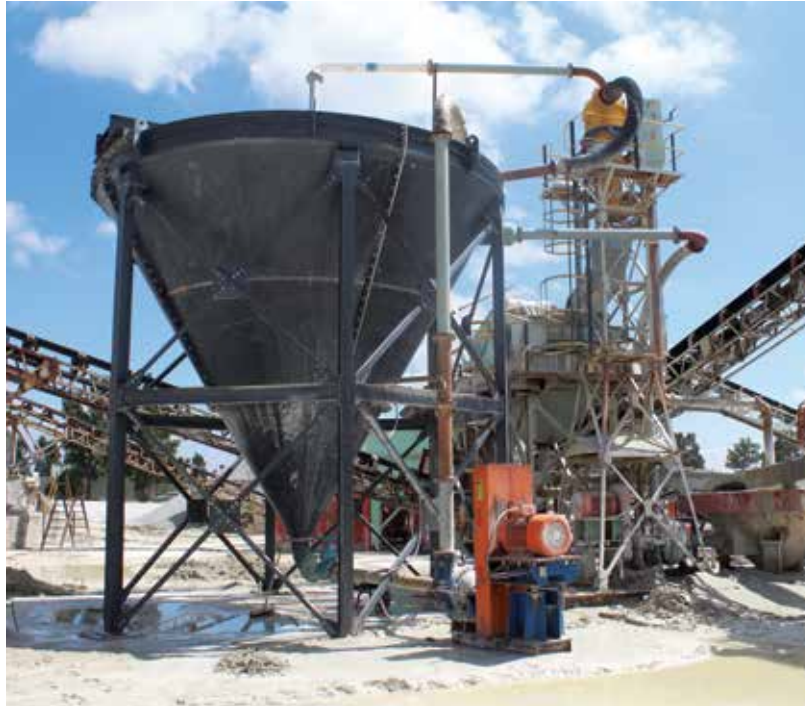
A larger dewatering cone (fines separator) was installed to recoup more sand.
