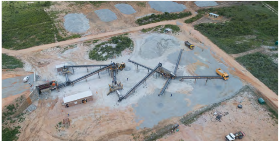
The scope of Osborn's contract for Beta Holdings included the manufacturing and supply of the equipment.
