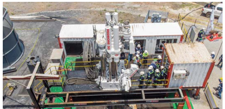
Redpath Thonket's record-breaking raiseboring work at the Obuasi Gold Mine in Ghana, featuring the Kwesi Mensah Ventilation Shaft – now the world's largest raisebore hole.
