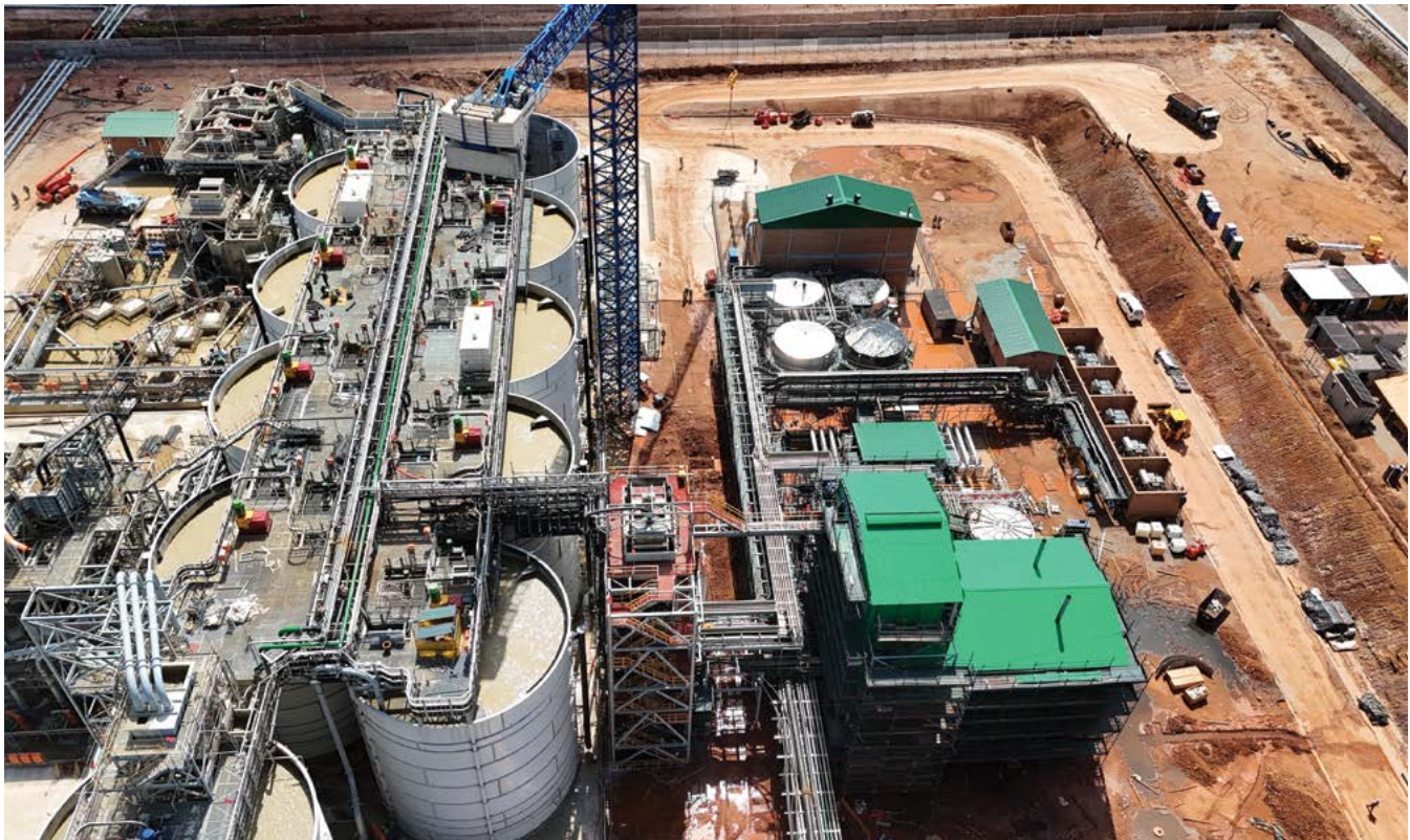
Processing plant CIL tanks.
