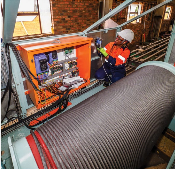
Tronox Mineral Sands has ordered a 35/12,5-ton Condra crane for mill maintenance.
