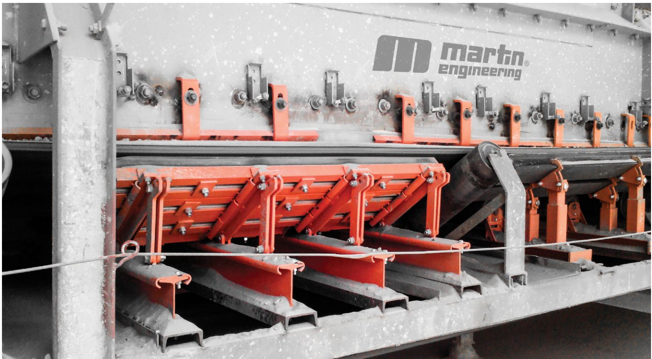
Raw material handling will never be 100% dust-free but good transfer point design can make it safe.
