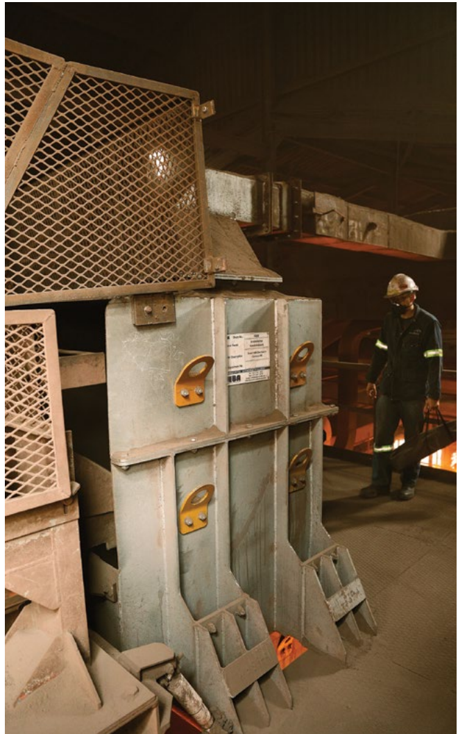
This Weba screen oversize-to-conveyor chute installation demonstrates how advanced flow control and sealing methods reduce dust, spillage and excessive wear at a steel plant.
