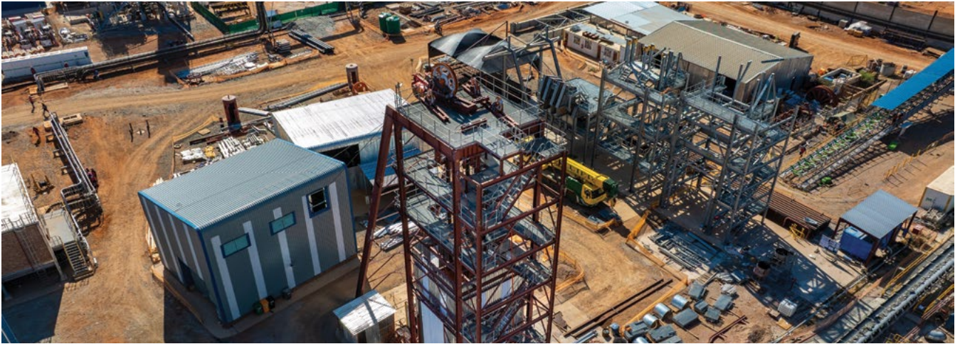
Work progresses at Platreef's Shaft #3, where Cementation Africa's pre-assembled permanent headgear can be seen to the right.
