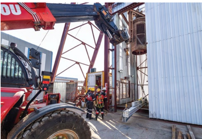
The Cementation Africa crew carries out precise slinging activities at Platreef's Shaft #3.
