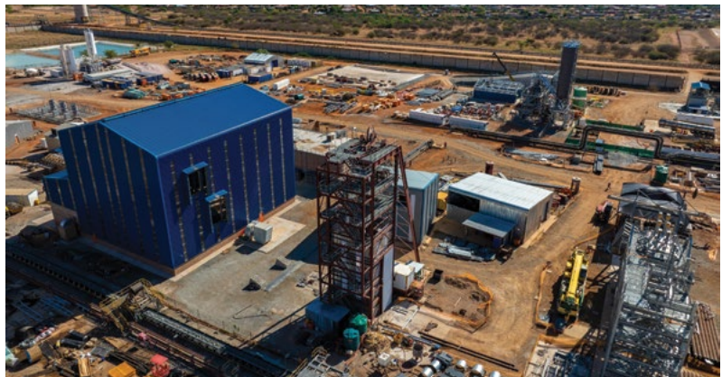
Platreef's Shaft #3 headgear, constructed by Cementation Africa, is shown alongside the permanent winder house on the left.
