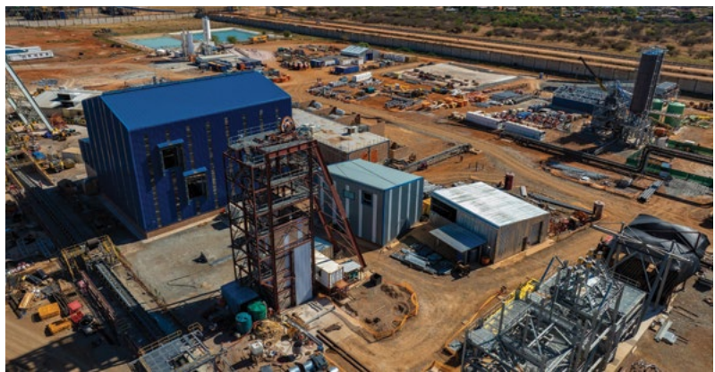
An aerial view captures Cementation Africa's progress on the equipping of Platreef's Shaft #3 head with both the stage and kibble winders in place.
