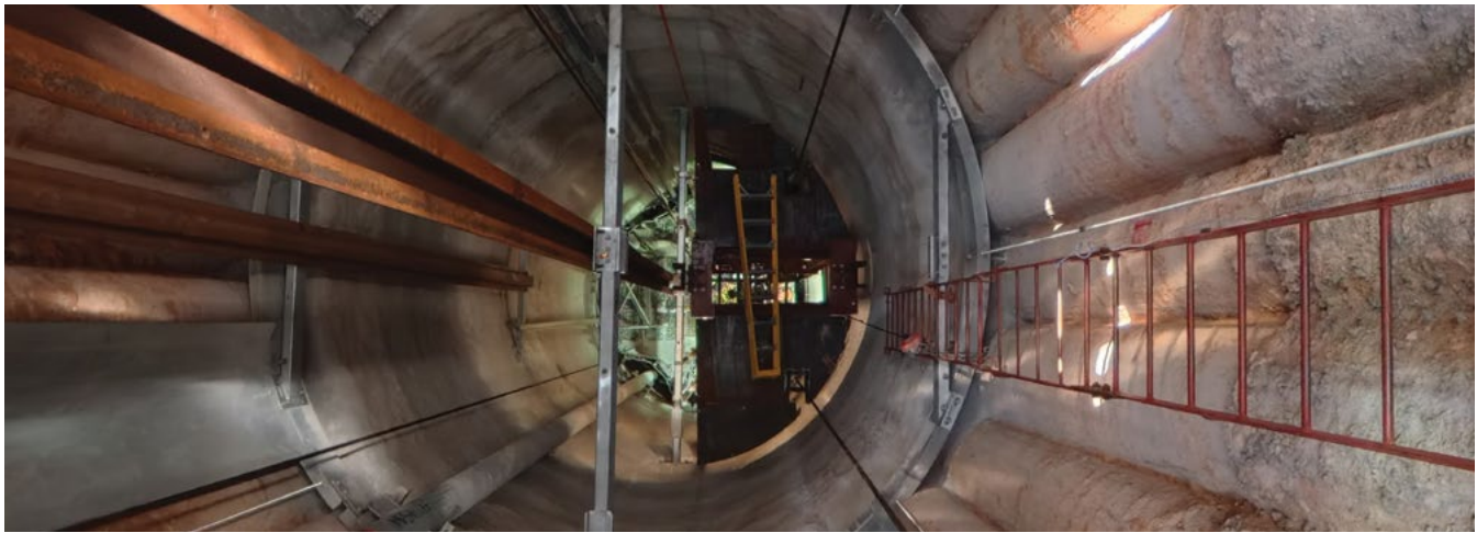
A view down into Platreef's Shaft #3 reveals Cementation Africa's detailed equipping process underway.
