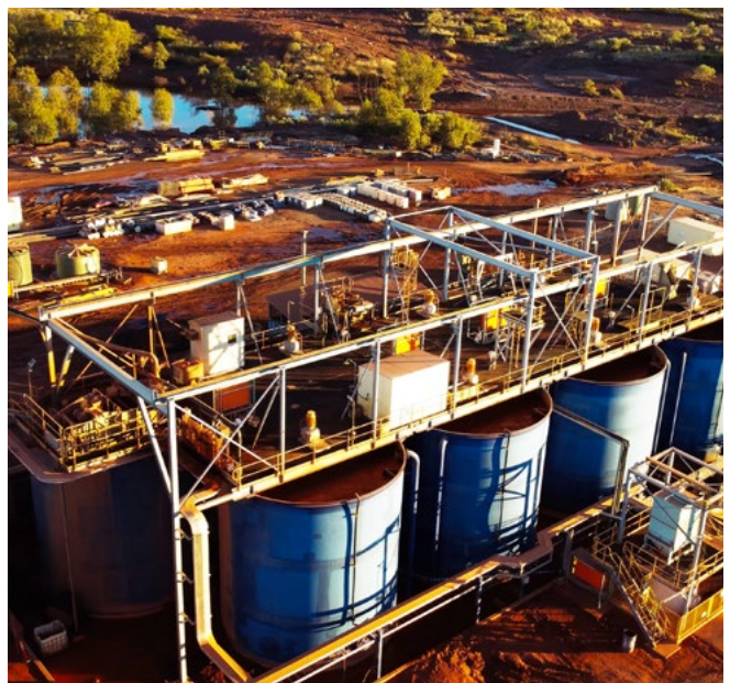
Tennant Mines successfully completed the construction of its 840 ktpa CIL gold processing plant at Nobles in April 2025.
