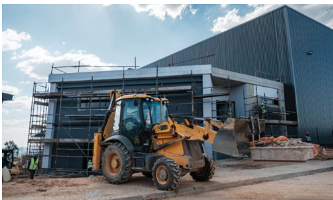
The impressive 17 000 m 2 SEW-EURODRIVE service and repair facility takes shape during construction, showcasing the scale of the company's latest investment in South Africa's industrial infrastructure.
