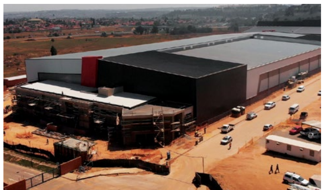
Purpose-built to OEM standards, the new SEW-EURODRIVE service and repair centre will bring all aspects of gearbox, motor and drive refurbishment under one roof - a first for the South African market.
