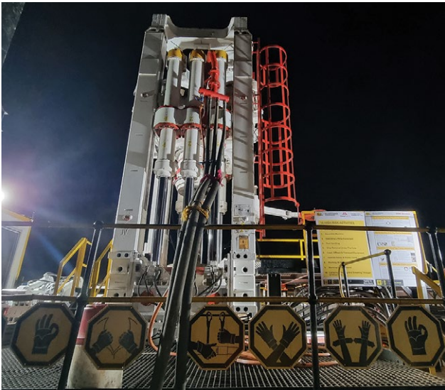
Murray & Roberts Cementation recently completed a 950 m borehole for a ventilation shaft at Ivanhoe Mines' Platreef Project.
