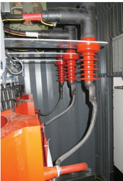
A dry-type transformer installed in modular substation.
