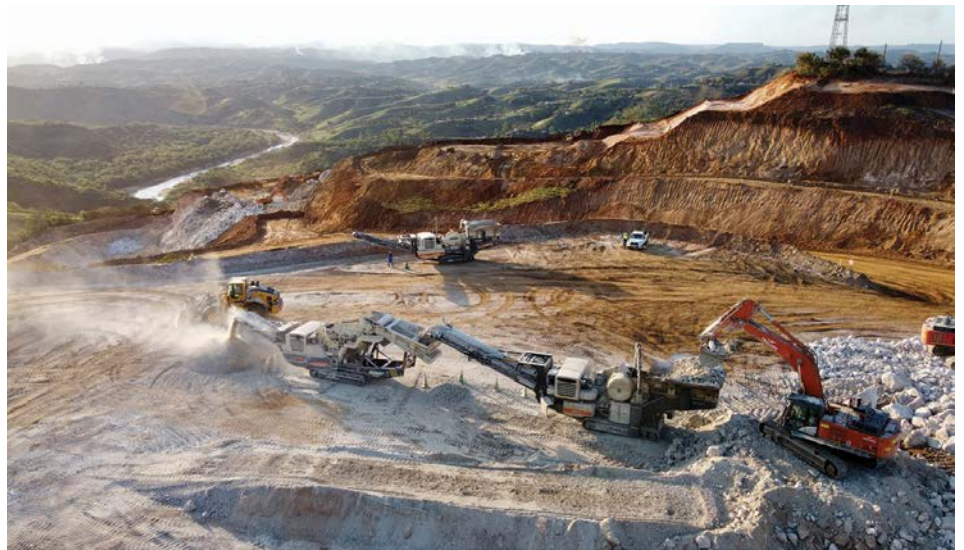
Overlooking the pit – the Metso mobile train processes primary and secondary crushing on-site.
