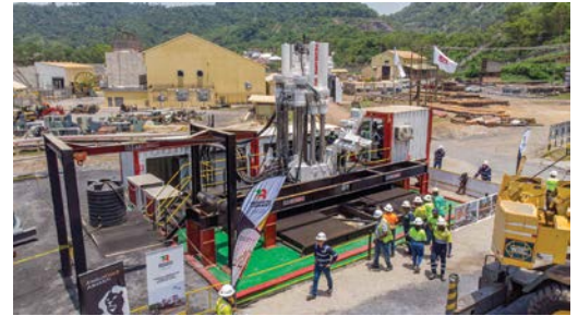
Guests and crew members gathered on 15 March 2024 to witness the holing of the Kwesi Mensah Ventilation Shaft.
