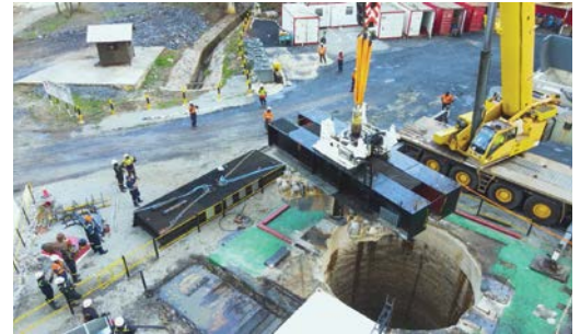
The Kwesi Mensah Ventilation Shaft - measuring in at a depth of 944 m and a diameter of 6.3 - 6.5 m.
