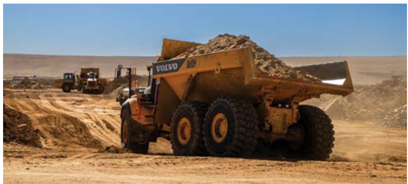
Yellow plant machinery started arriving at Gugulethu Colliery in the first six months of development.
