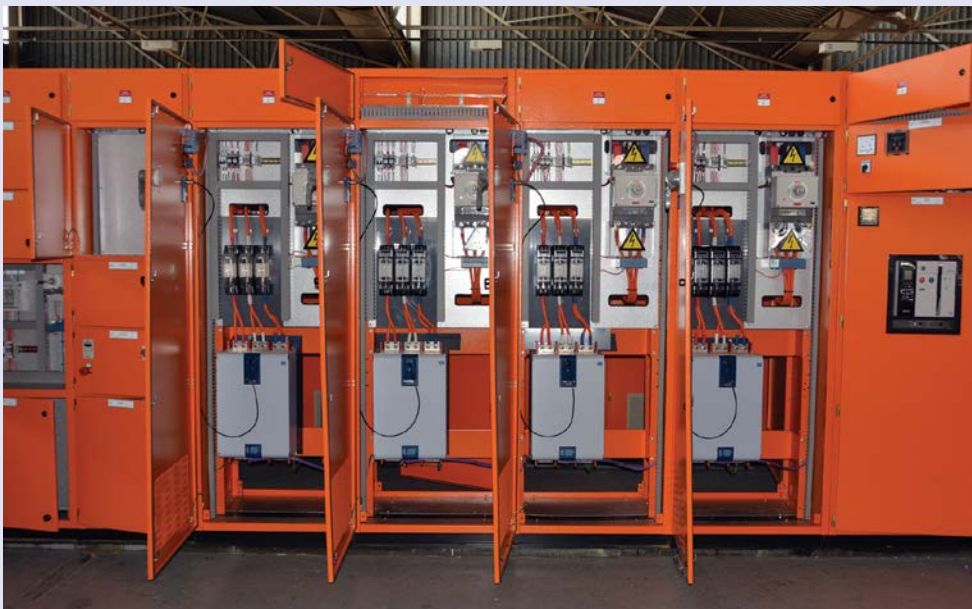
Low voltage variable speed drives in a motor control centre.
