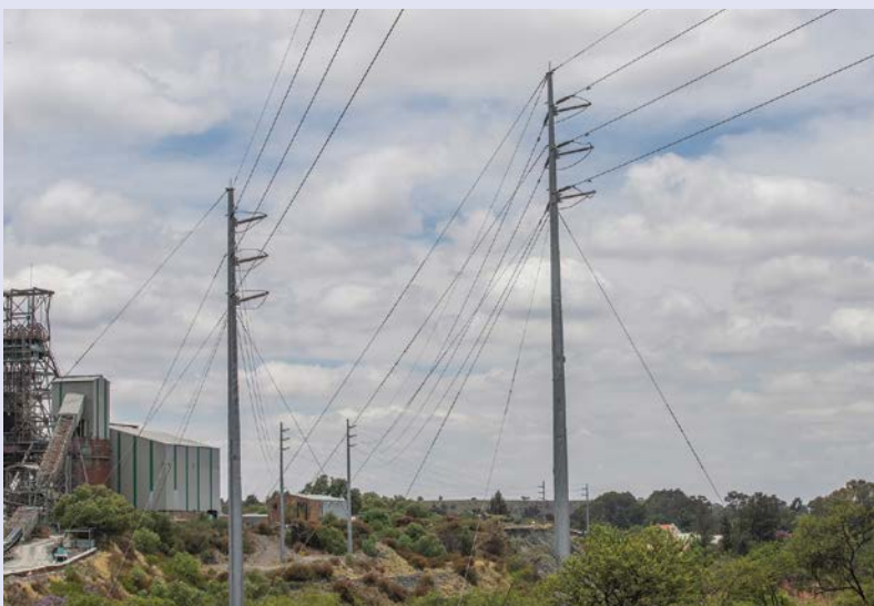
Overhead cables running power into a mine.
