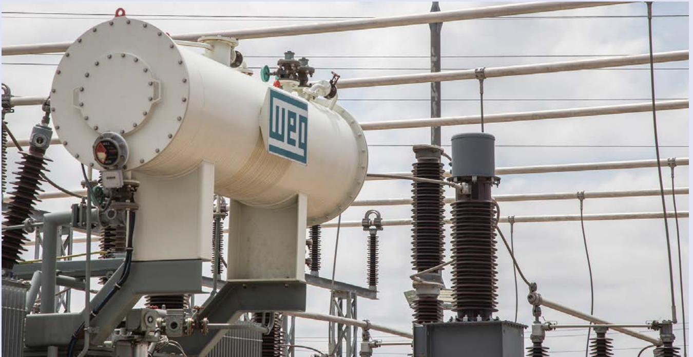
WEG transformer distributing power into a mine's operations.
