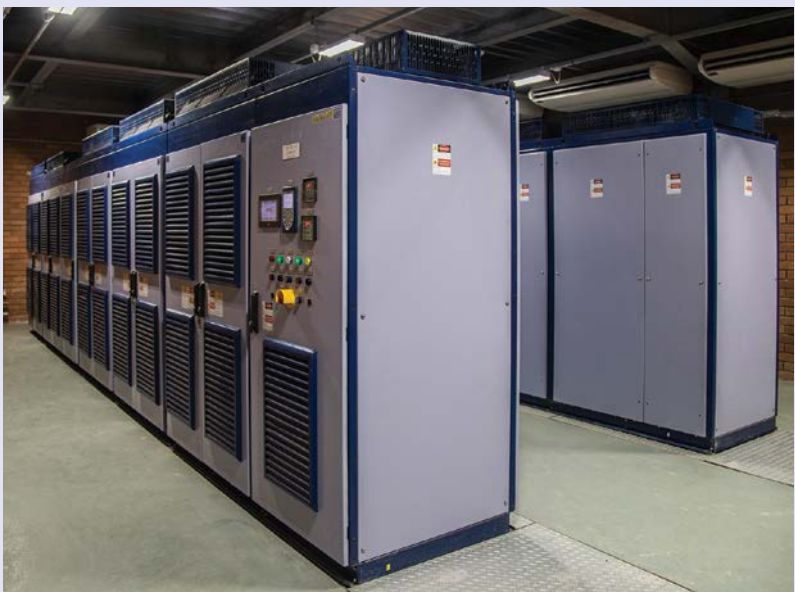
WEG medium voltage variable speed drives operating in a mine.
