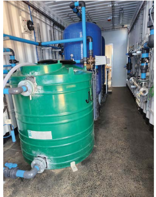
Feed tank to supply softening process (PWTP). This is post-filtration through the sediment and granular activated carbon filters (shown in background – blue vessels).
