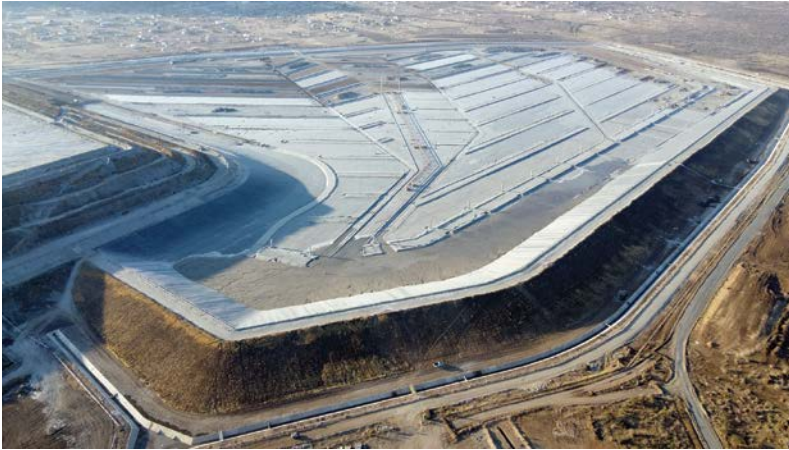
The GISTM requires that factors like climate change be considered in the design of tailings dams.
