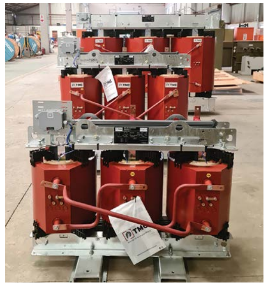
These three specialised dry-type transformers were supplied to a gold mine.
