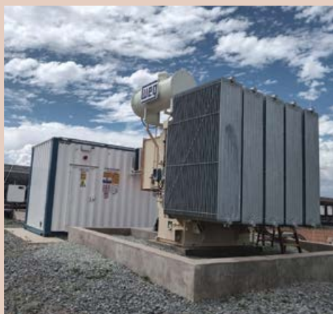
Zest WEG manufactures transformers for the solar industry.
