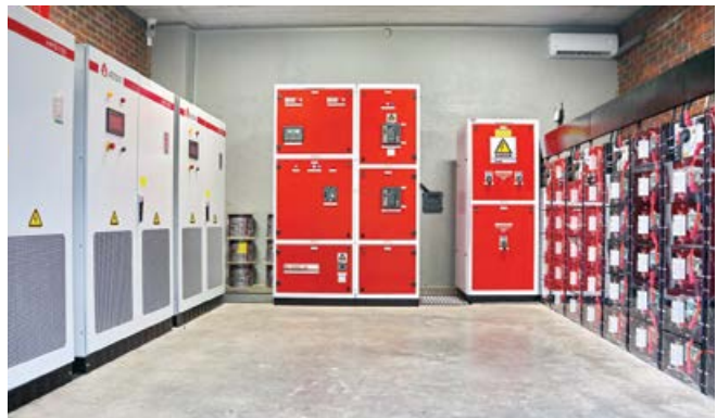
A view of the solar room used to power the Brelko factory.
