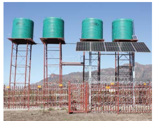
A view of the water tanks.
