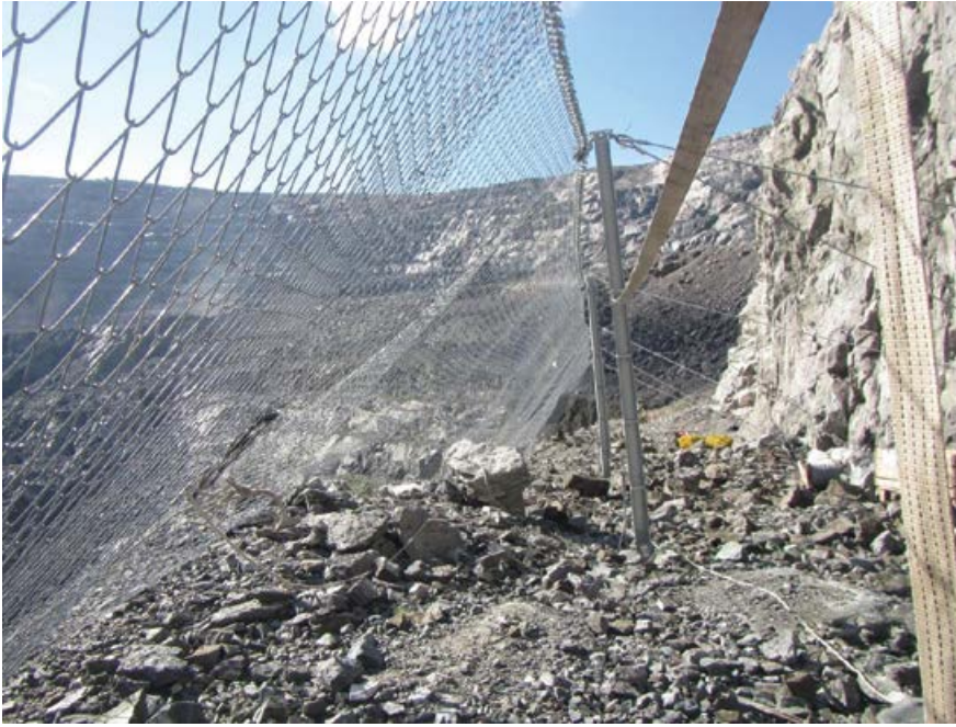
Attenuator at local diamond mine.
