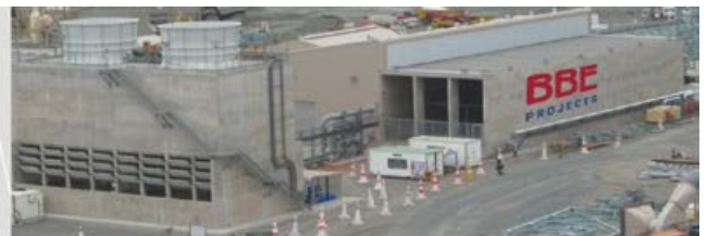
Photo: Refrigeration plant and bulk air cooler, Venetia
