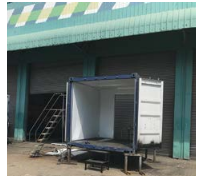
3 m containers in the process of being converted into substations.
