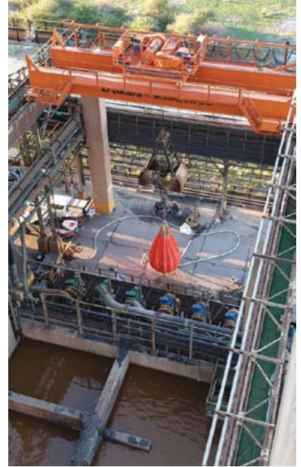
Crane automation is the most noticeable trend in Africa's overhead crane industry.
