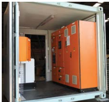
A 3 m container converted into a substation and equipped with LV MCC and DB plus MV incomer switchgear.
