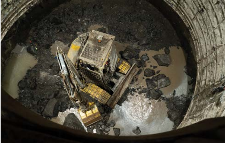
An excavator busy lashing at the shaft bottom with shaft lining being carried out on the face.
