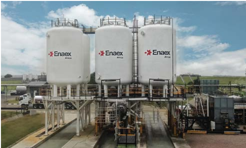
Bulk Emulsions plant in Secunda.
