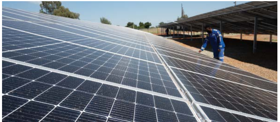
There are more than 9 GW of renewable energy projects that can be built in the next five years.
