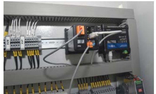
Installed V-CUBE at client site.
