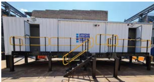
The E-house at the manufacturing facility in South Africa.
