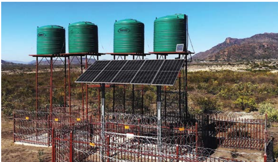
Nkwe Platinum rolls-out solar-powered water system for the community.
