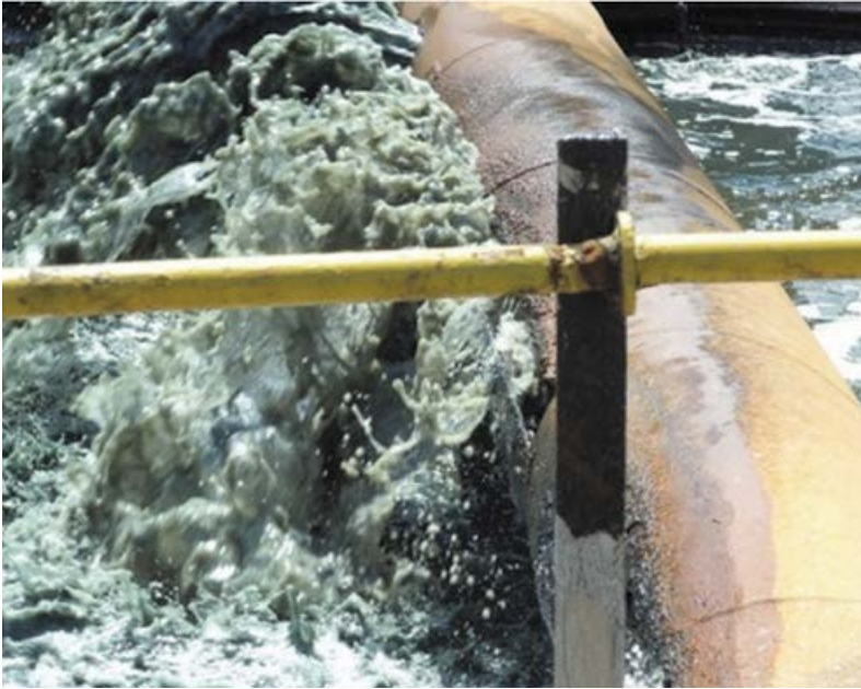
AMD treatment plant in the West Rand.
