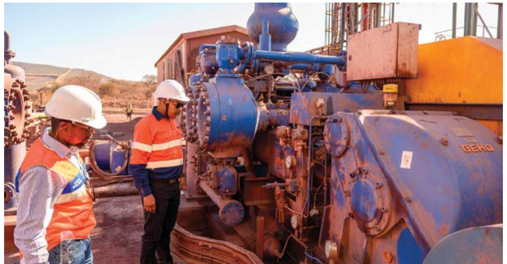
Weir Minerals' GEHO positive displacement pump installed in the tailings section at a fluorspar application.
