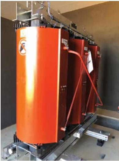
A 3150 kVA 11 kV/400 V cast resin transformer for a mining-specific application, installed in an indoor substation.
