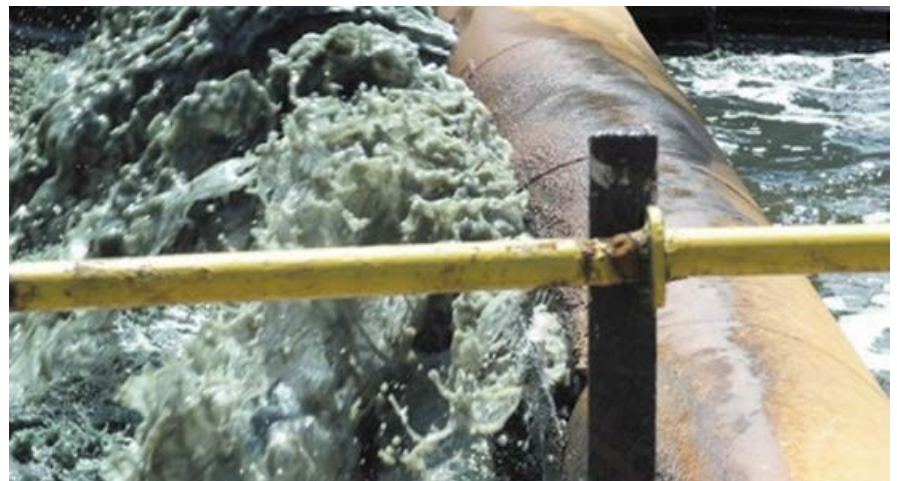
The Eastern Basin AMD plant has not been able to treat acid mine water since February 2022 owing to failure of pump motors.
