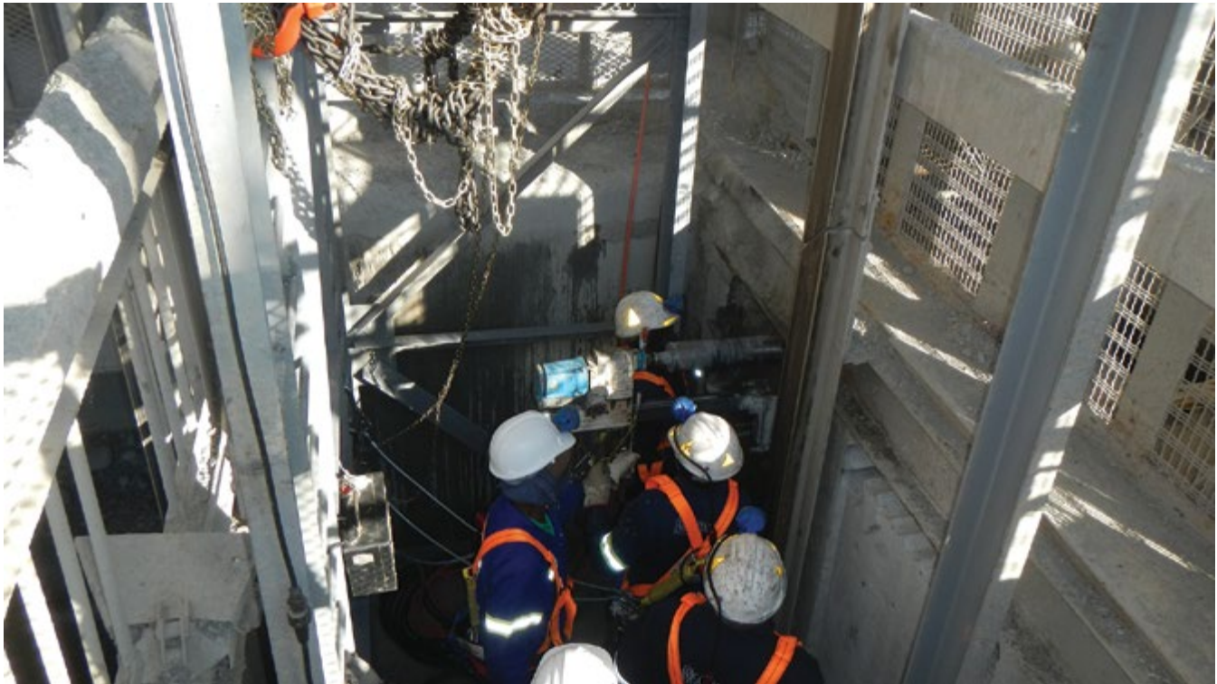
Cutting the wall also proved to be a challenge as it was very old and had no reinforced steel.
