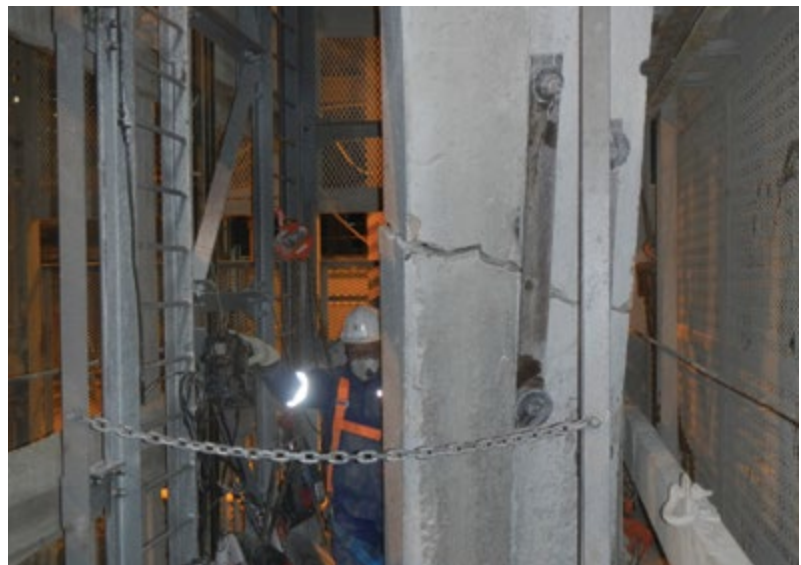
A portion of the brattice wall in the shaft had to be cut from the surface down to 9 m below.
