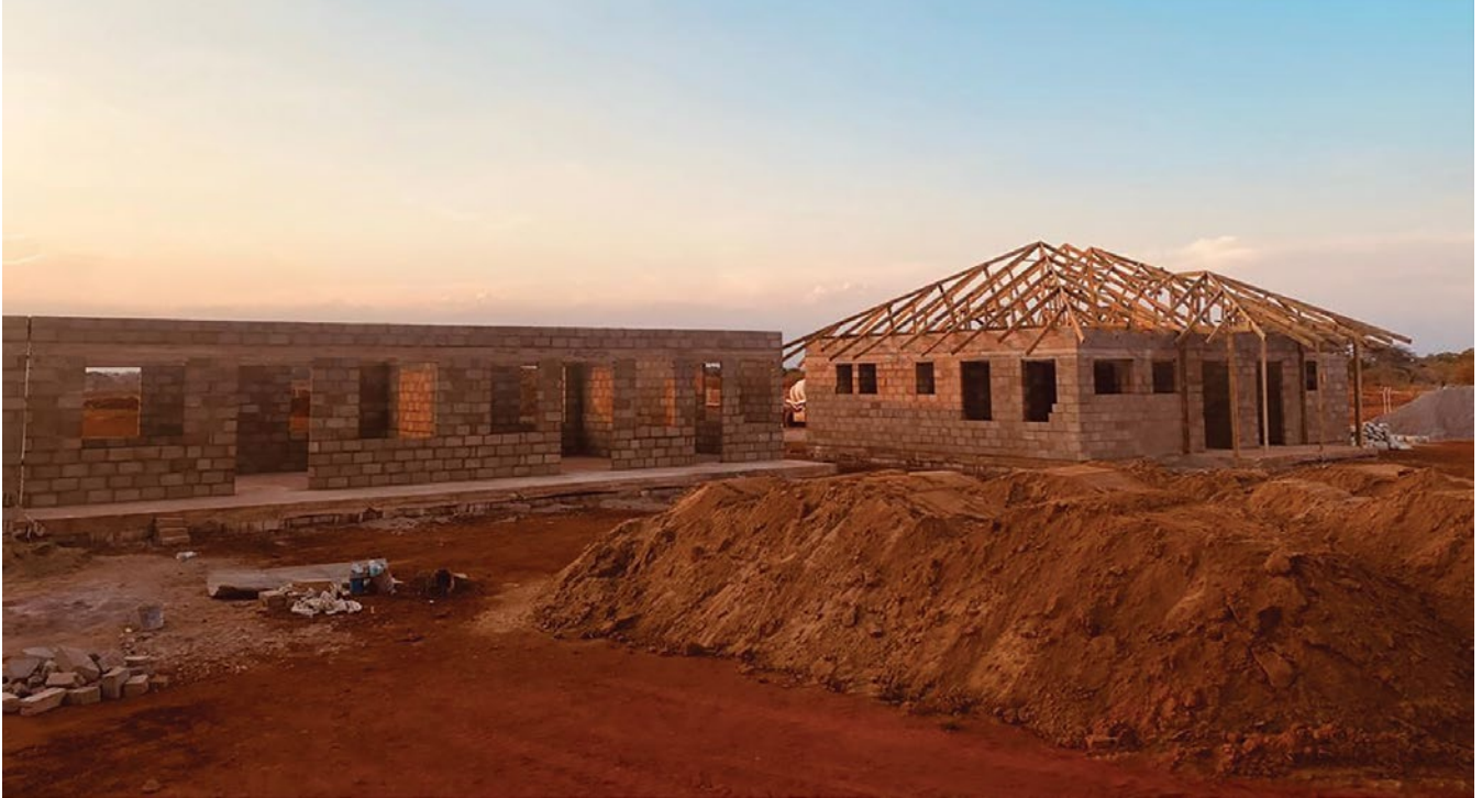
Key infrastructure such as bulk power, water and buildings are progressing on track.
