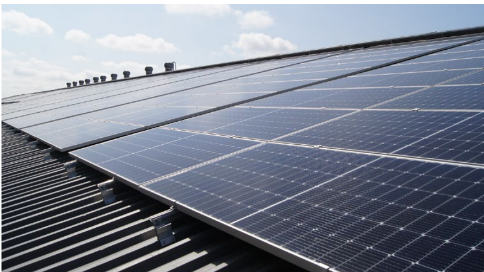
Astec AME has made a significant investment in a solar energy plant at its Astec Johannesburg manufacturing facility.
