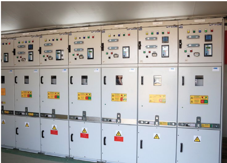
Zest WEG supplied a locally manufactured MTW05 Medium Voltage switchboard to a gold producer in Gauteng.
