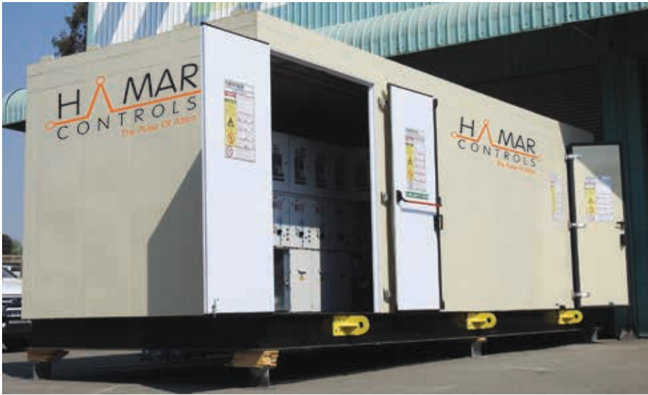
Hamar Controls' newly-built mobile electric substation destined for Mozambique.
