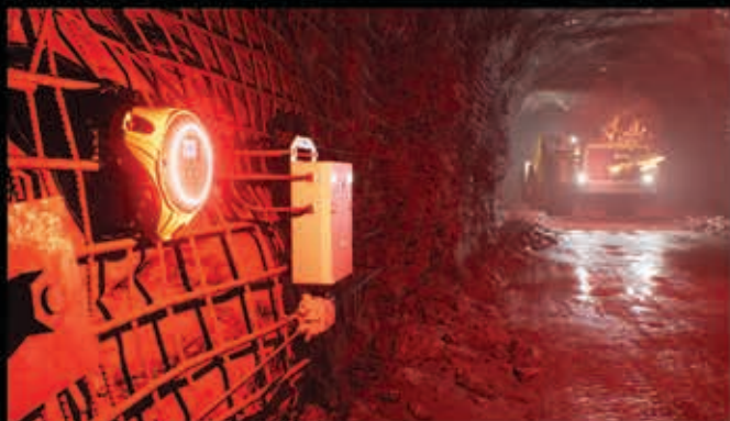
SITE-WIDE GAS MONITORING
