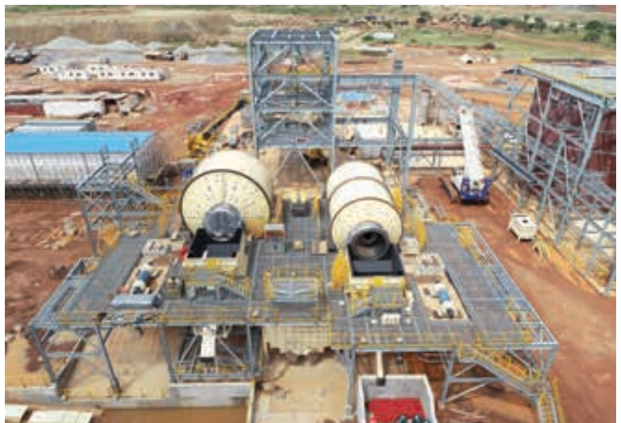
The SAG and ball mill components are on site and partially erected (photo: West African Resources).
