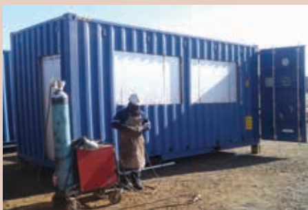
WEG Automation Africa has supplied a containerised substation and control room solution for a tin mine in the DRC.
