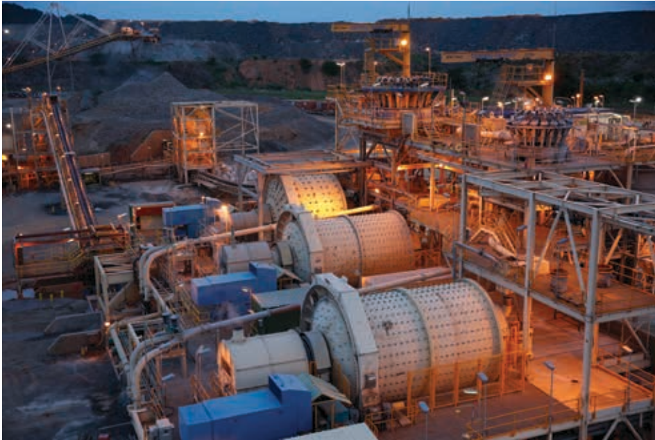
It is envisaged that the Sabodala processing plant, seen here, will treat ore from Massawa (photo: Teranga).
