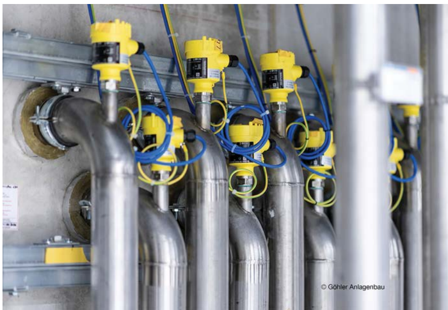
The new chemical tank farm at Scharr is equipped with around 170 VEGASWING 63 vibrating level switches, which protect the tanks from overfilling and leaks.
