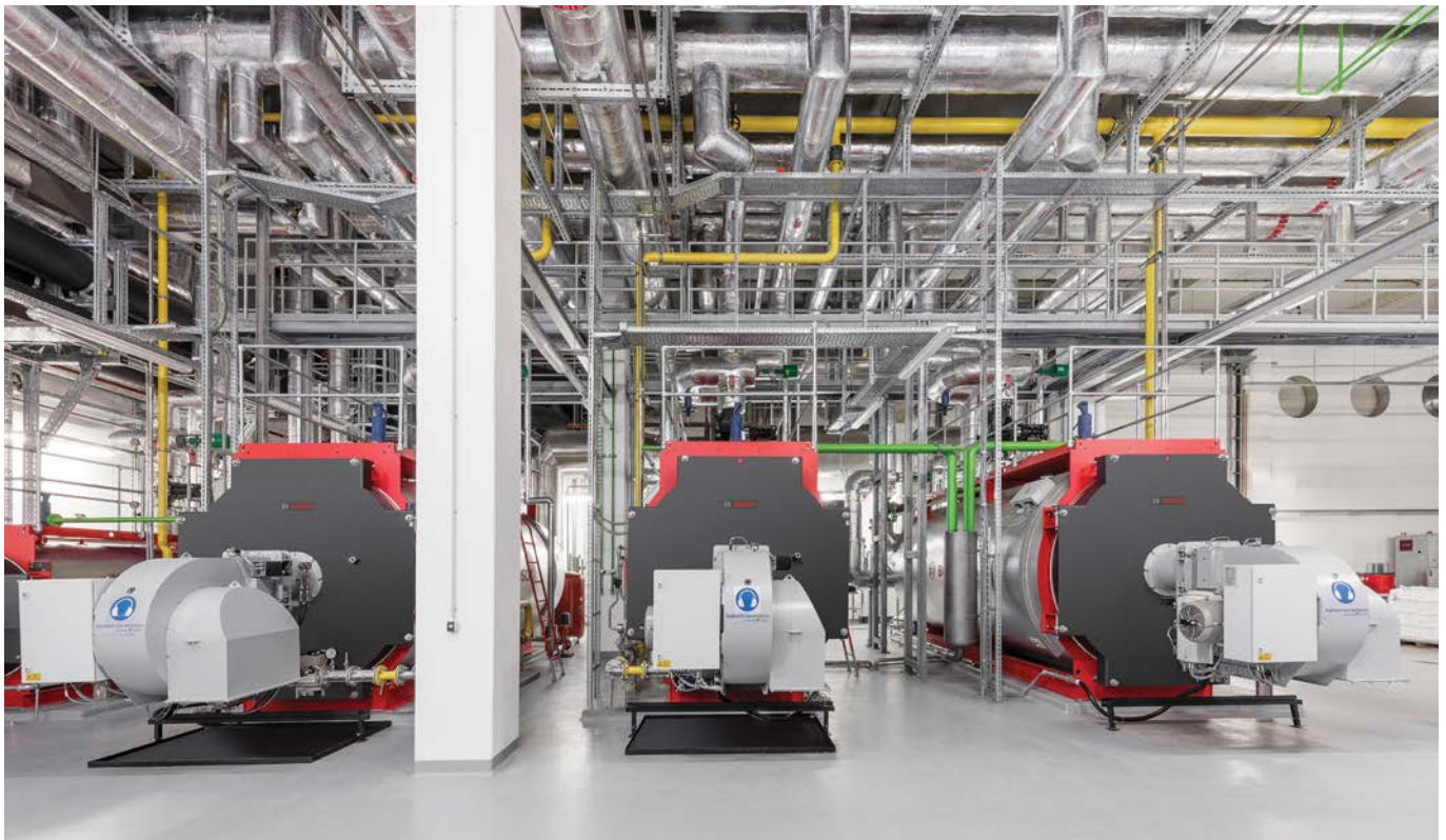
The Robert Bosch GmbH Research and Development (R&D) centre in Schwieberdingen, Germany, develops advanced energy solutions from traditional industrial boilers to future-proofed, decentralised systems.
