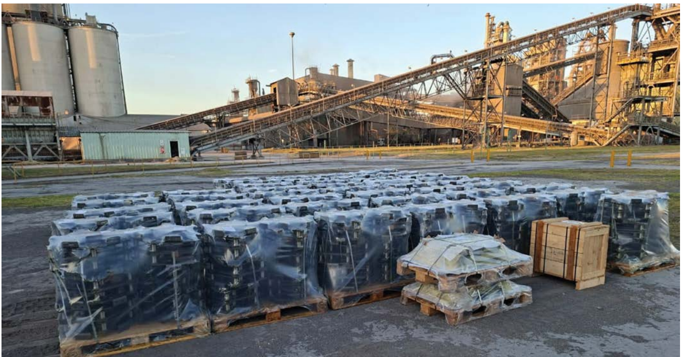
Bi recently installed a high-performance Kobo dual/double-chain pan conveyor in the cement industry, a first-of-its-kind installation in South Africa. Kobo heavy-duty chains can enhance reliability, efficiency and longevity.
