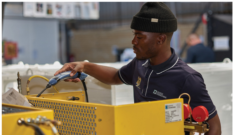
In a demanding underground mine in India, Booyco Engineering's HVAC system operates up to 20 hours a day in high heat and humidity.
