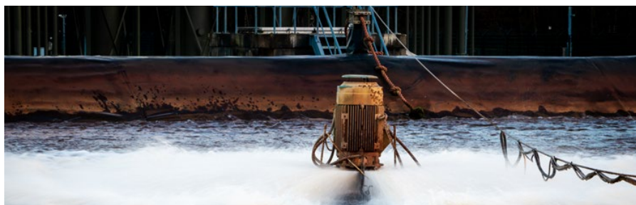
"We need to better manage our scarce water resources sustainably with infrastructure that is fit for purpose," says Obermeyer.
