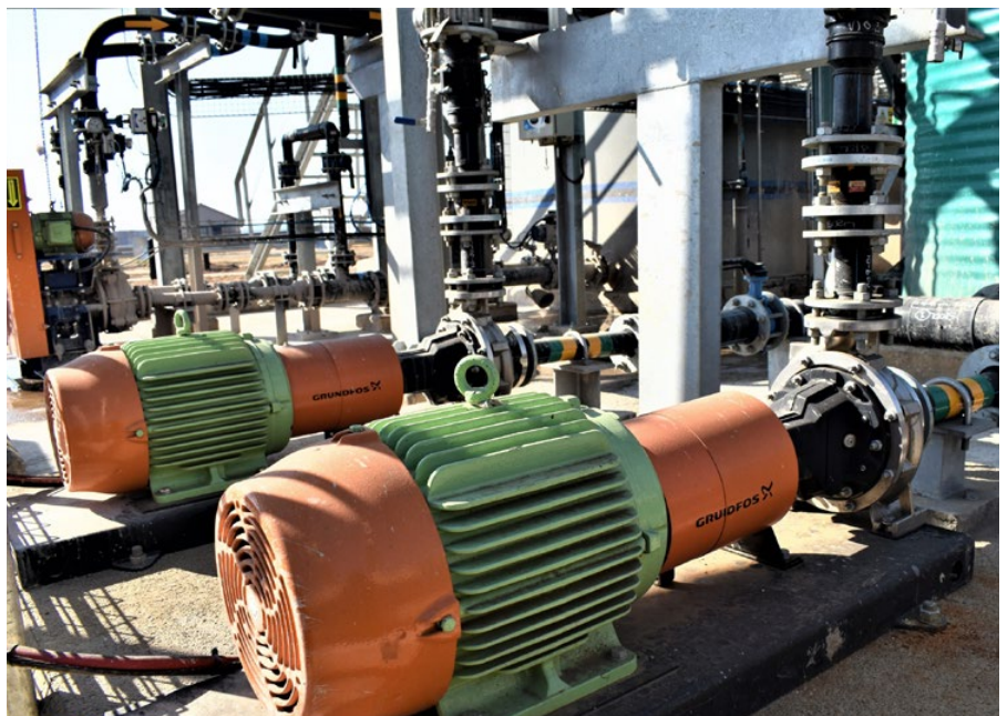
Grundfos booster pumps for pumping water from the permeate water tank to the slaker tank and for backwash.
