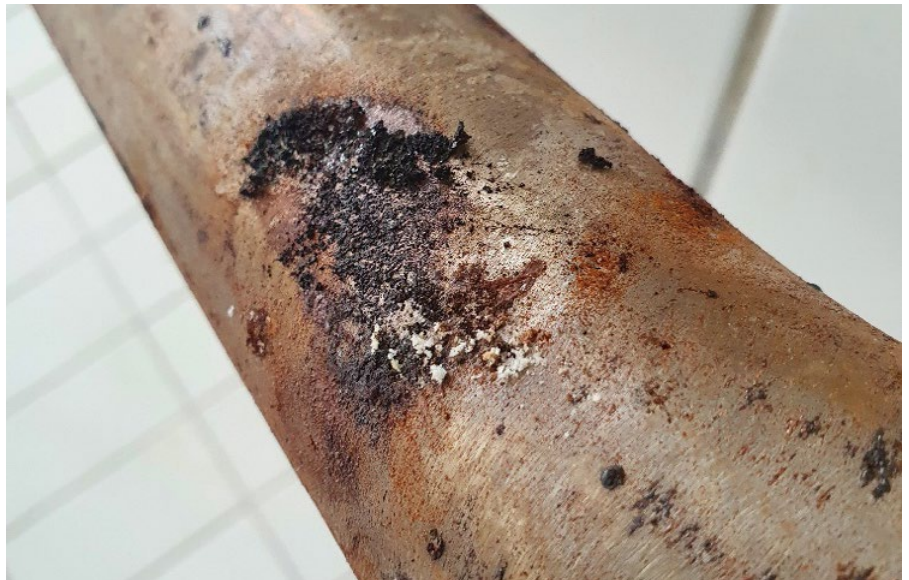
Figure 2: Damage to the material surface caused by pitting corrosion. At the lower right, a very rough surface finish is visible, while on the right, the mounting to the pool structure reveals the onset of crevice corrosion.
