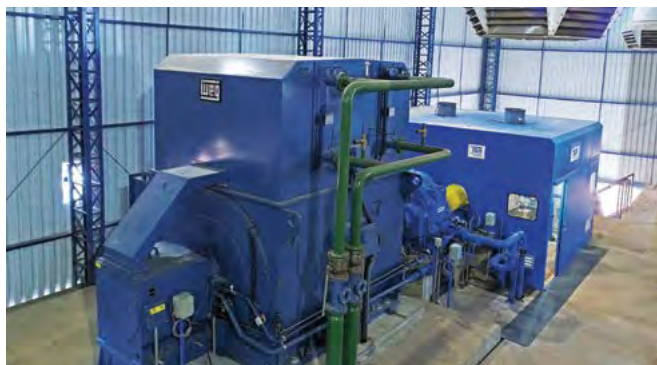
A backpressure turbine generator for a sugar mill.
