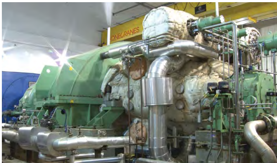
A condensing extraction turbine generator at a paper mill, which enables condensed steam to be recirculated as boiler feed water.
