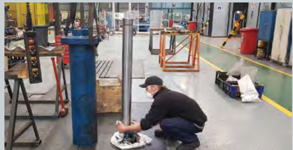
The cylinder repair work was executed during South Africa’s national COVID-19 lockdown to minimise downtime at the plant.
