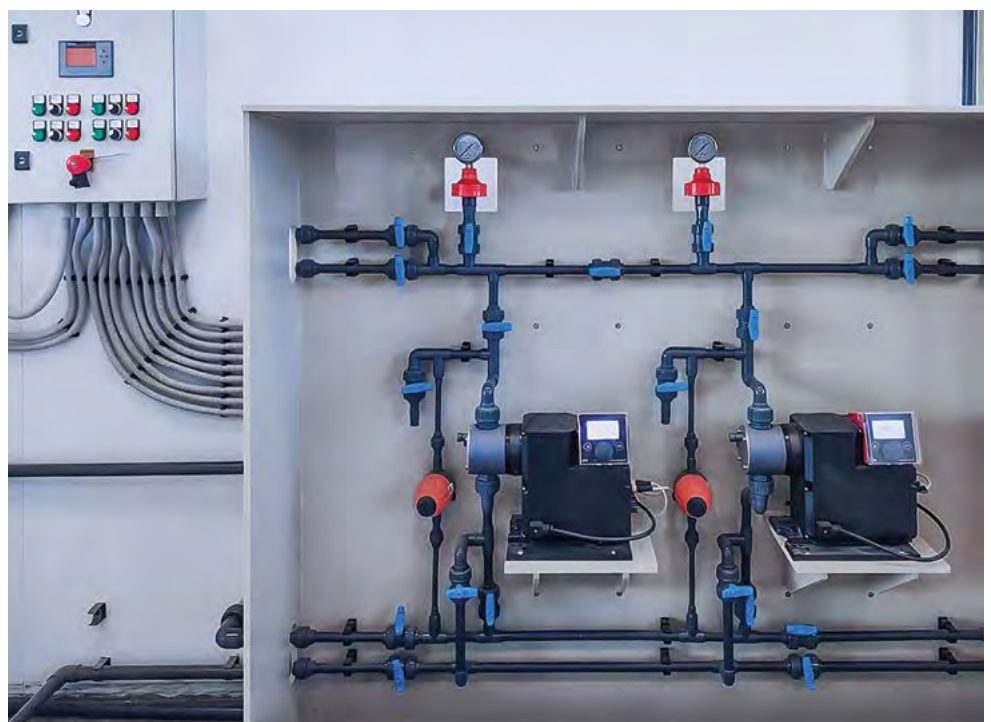
A close-up view of Grundfos Smart digital XL dosing pumps like the ones being used at the Nootgedacht Water Treatment Plant.
