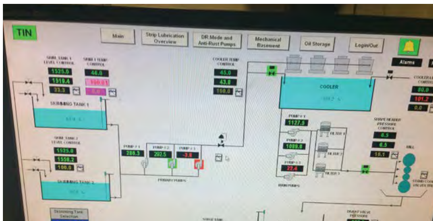
Accessing information remotely is all part of the modern plant's infrastructure. SCADA or DCS systems can be accessed from home or during online training.
