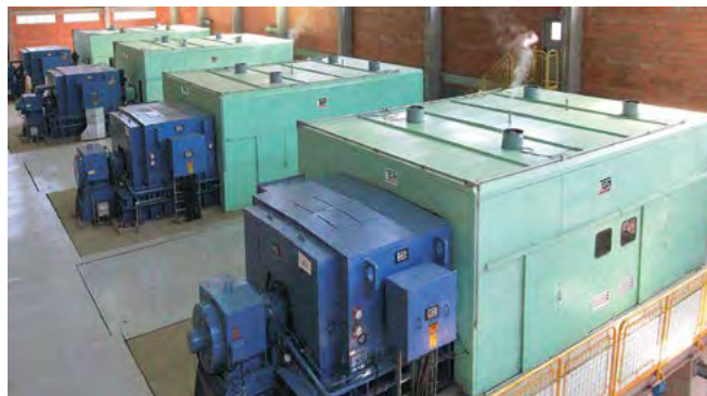
TGM WEG steam turbine generator sets at a sugar mill.
