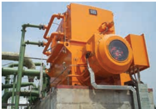
A WEG-wound rotor induction motor installed on site.
