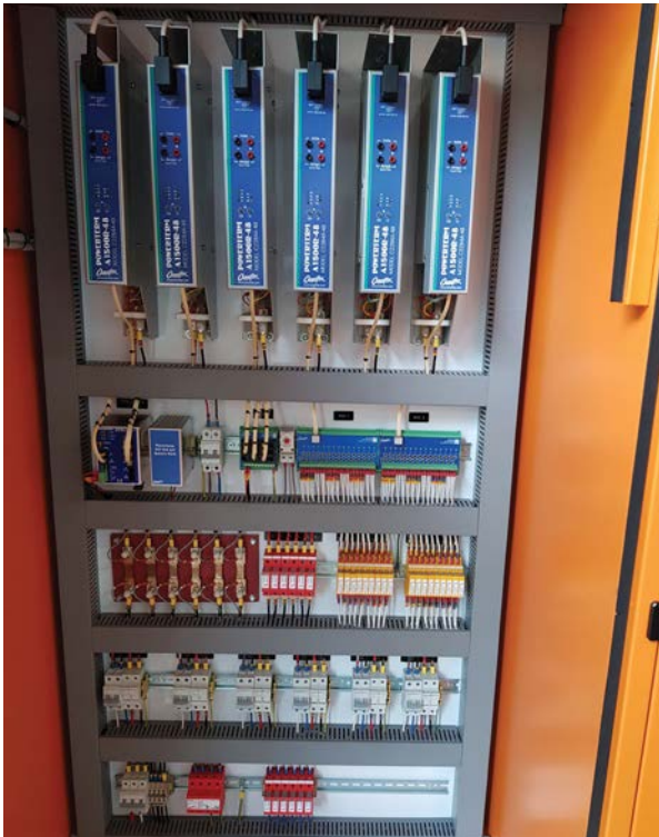
Remote monitoring can transform performance and safety in bulk fuel storage tanks.
