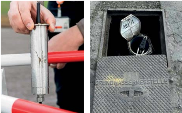
Left: Keller Data Logger ADT1. Right: Keller groundwater measuring installation.
